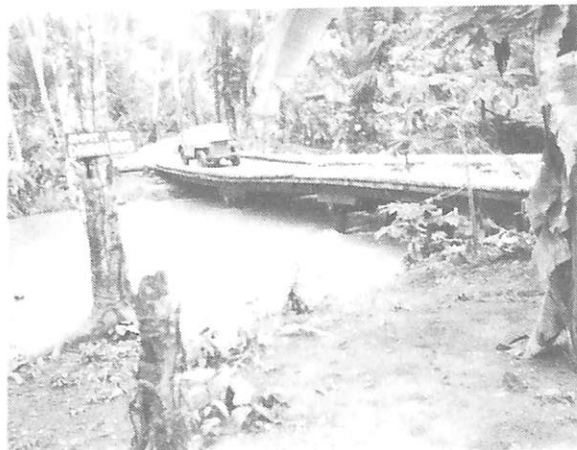
Milne Bay. Normal coconut bridge sagging after flood which at one time was over the bridge. (Author's collection)
